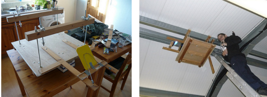
Fig. 3. Phase 1, (left) projector platform being constructed, note mirror cantilevered from the platform, and (right) installation at 5m apex of Rural Centre roof.
